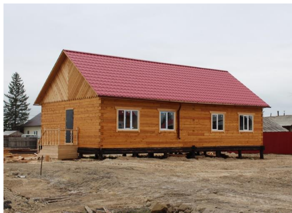
Fig. 39. Adaptation of construction technology to the conditions of permafrost degradation: building a house on a pile foundation, Amga, September 2022. Photo by S.A. Grigoryev.
