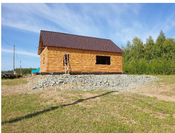
Fig. 40. Adaptation of construction technology to the conditions of permafrost degradation: building a house on a bedrock fill and a metal frame as a foundation, Ulakhan-An, August 2022. Photo by A.A. Suleymanov.
