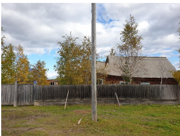
Fig. 14. One of the houses affected by thermokarst. A new house, to which the owners of the site were forced to move, is in the background on the left, Yunkyur, September 2022. Photo by A.A. Suleymanov.
