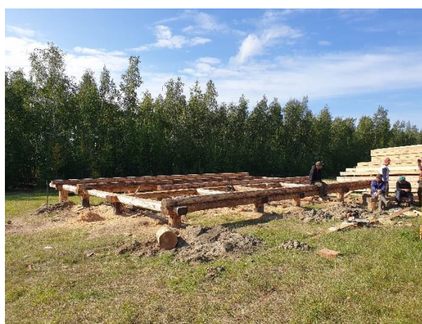
Fig. 41. Adaptation of construction technology to the conditions of permafrost degradation: construction of house foundation on 5-metre larch piles, Ulakhan-An, August 2022. Photo by A.A. Suleymanov.
